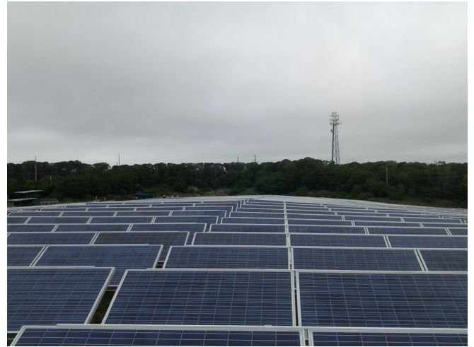
Orleans Capped Landfill Solar PV
